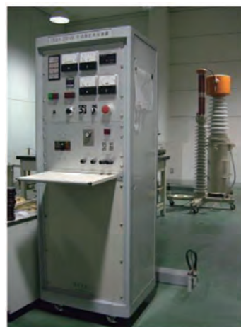
Fig. 2 High voltage generator.
