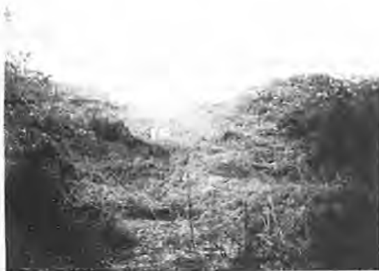
図7 崩壊斜面 Failed Slope
